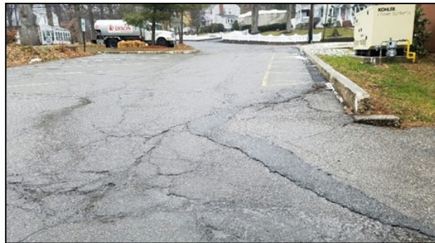
View of deterioration to the Senior Center parking lot. Grant-funded construction, commencing in May, will provide for necessary repairs.
